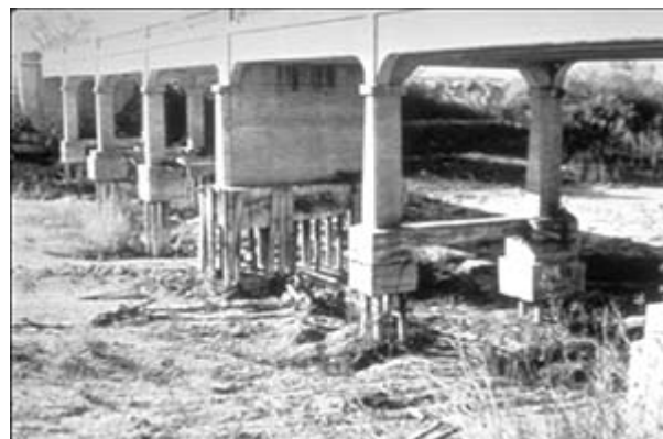
Figure 5-33 Effects of Bridge Scour
