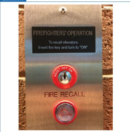
Elevator lobby emergency operations key switch.
