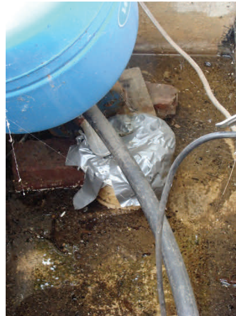
Example of an improper repair: water well with duct tape used as a sanitary seal.
